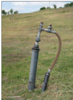
Gas extraction well
