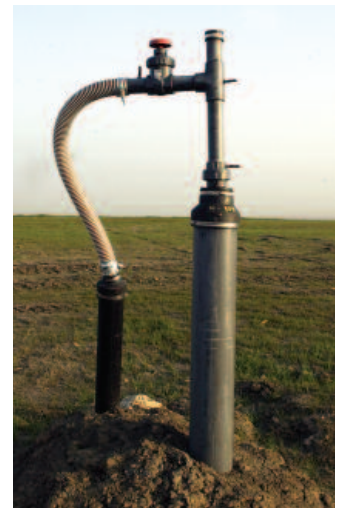
Gas extraction well
